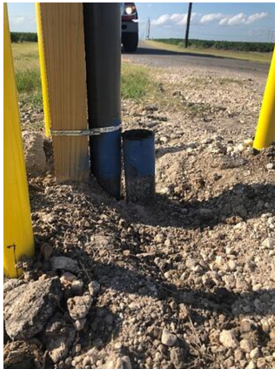
Figure 4. Low-Side Casing Vent Pipe- Clearance and Obstruction Issues.
